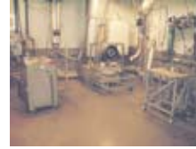
Pneumatic Test Cell #7
