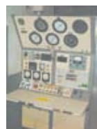
Pneumatic Test Cell #4
